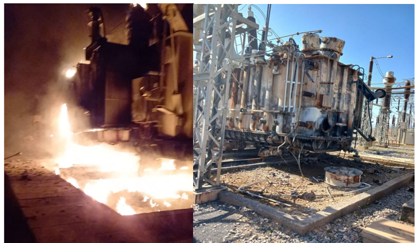
Figure 6. Fire at the Tekeze substation due to drone attack (own photograph in the aftermath of the attack).
